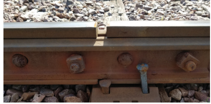
Gap Too Wide
