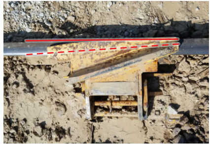
Not Properly Aligned with Rail
