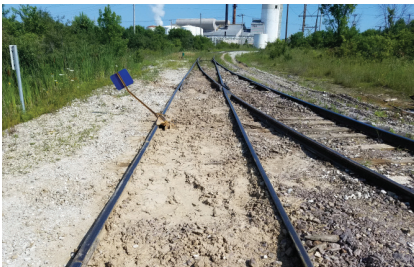
Muddy Track Ballast
