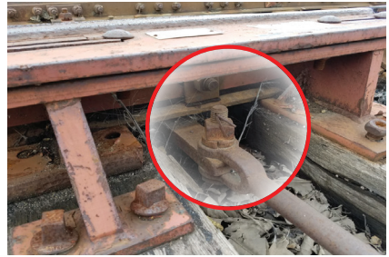
Rod Bolt at Track
