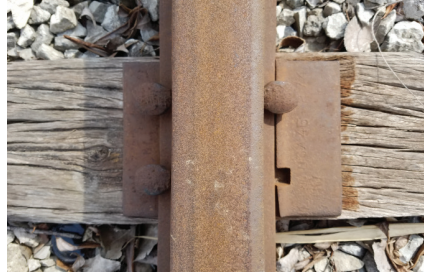
Tie Plate Rubbing on Tie
