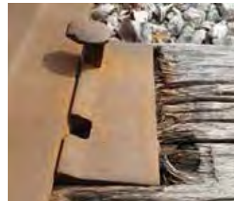
Lifted spikes between the rails
