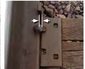
Rail base and tie plate gap
